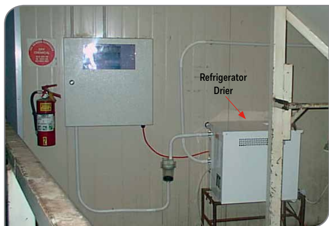
Figure 4 - ASD with refrigerator drier
